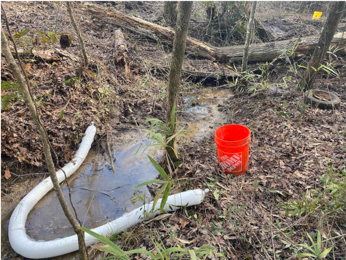
Kiel on the scene in Greenville, Al. recovering a spill of non-hazardous epoxy resin from a tanker rollover. Nice work, Kiel!
